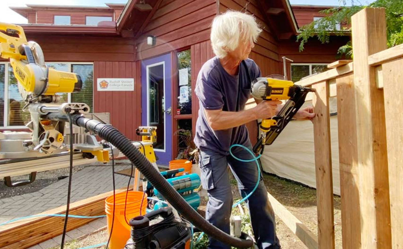
Vadim Guitman from TWS installs a new fence along the east side of the Rudolf Steiner College Canada courtyard.
